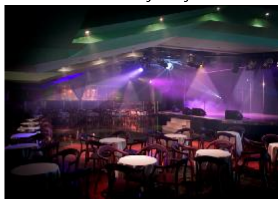
Modern lighting system
